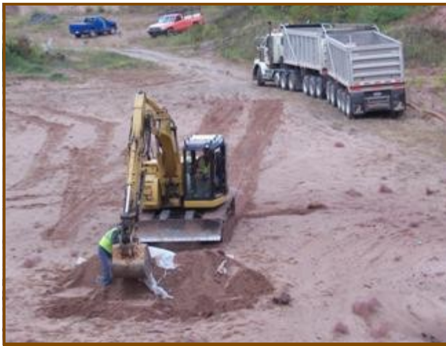
Excavation of contaminated soil at the sand pit on Indian Cemetery Road.
