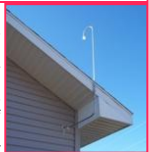
Ozone air intake and ventilation
